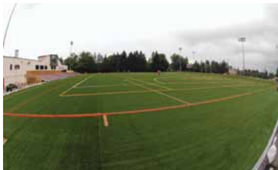
The renovation of North Country Field, with Hall-Leet Stadium under construction to the left, proceeded through the summer.
